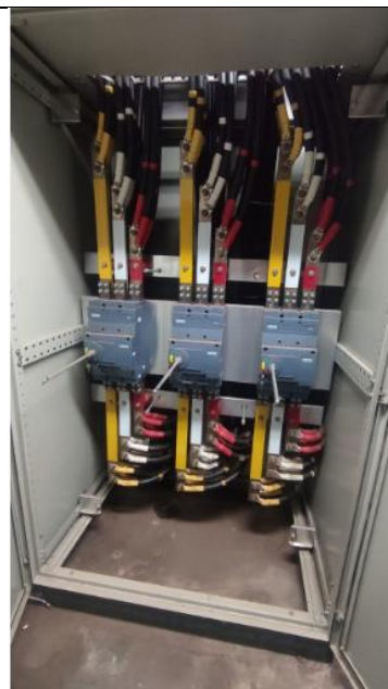
8. QDG Trafos 2000x1200x850 porta dupla
